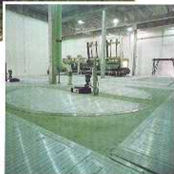
Pictured above: In the treatment plant's headworks building, covers for the grit chambers and effluent channels require interlocking panels that are complex and difficult to fit.
