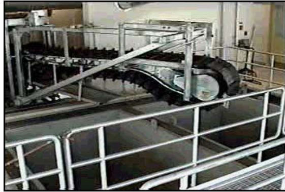
Serpentix P2 conveyor with a flex-end discharge at work in a water treatment facility
