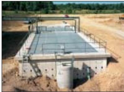
"It's working great...I have no complaints," said Jerry Schwarts, plant operator, referring to Chapman's new Fluidyne ISAM™ system, shown here during installation.
