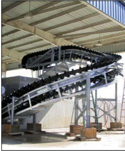
In tight quarters, a P2 Pathwinder makes a 180 degree helical turn.
