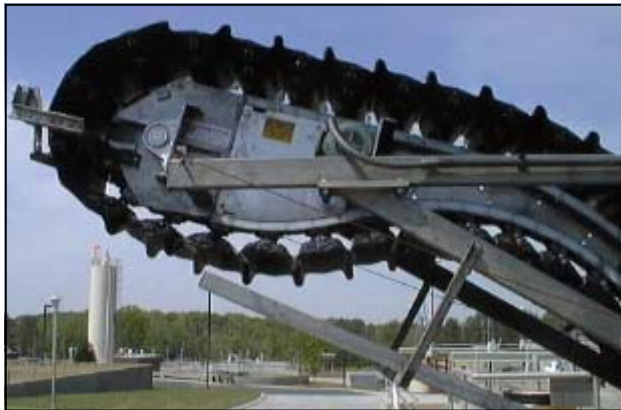
A P2 drive structure with scraper bar. This conveyor hauls grit and screenings collected from the inflow channel of a wastewater treatment plant.
